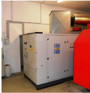
CHP of 150 kWel in Hotel Mons in Slovenia (source: Code2)
